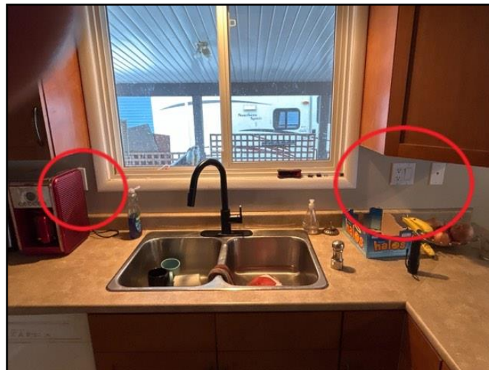
GFCI plugs missing
