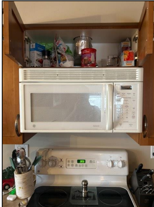
Exhaust fan discharges to the exterior
