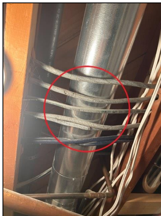
Wires touching ducts
