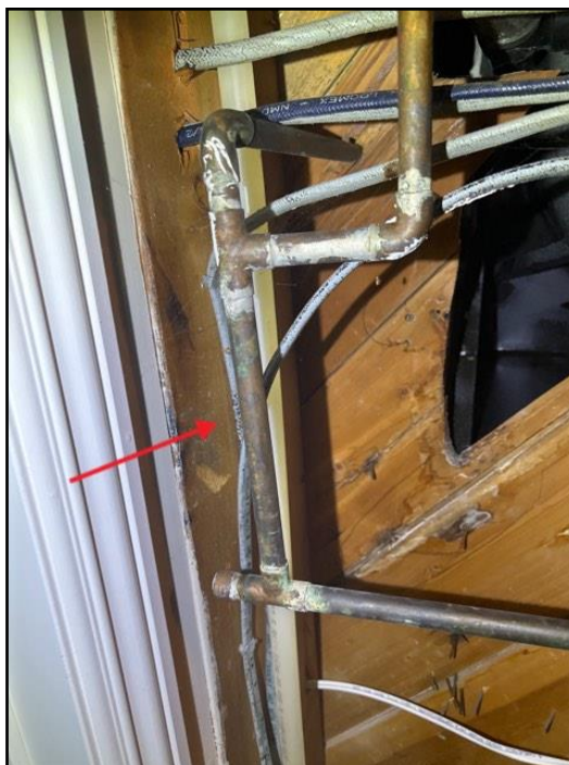
Old copper pipes
