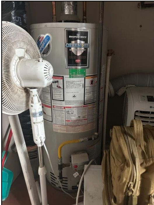
Conventional water heater
