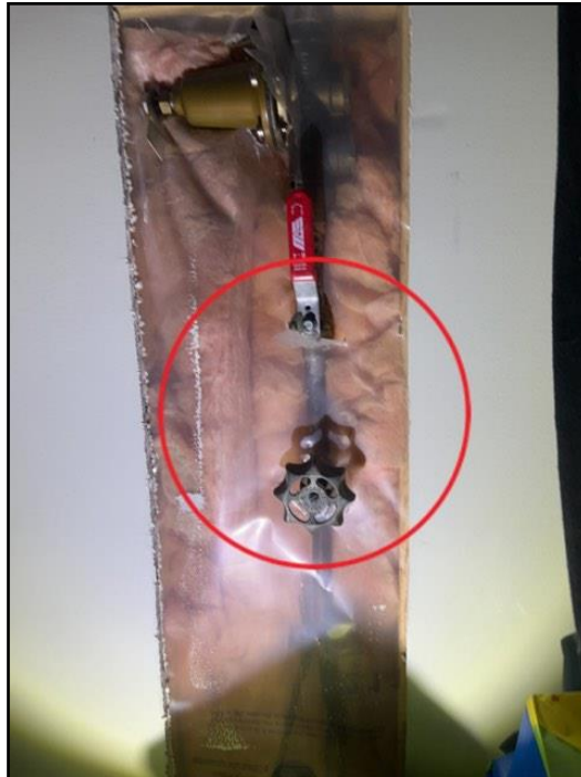
Water shut off
