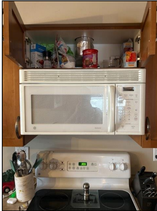
Exhaust fan discharges to the exterior
