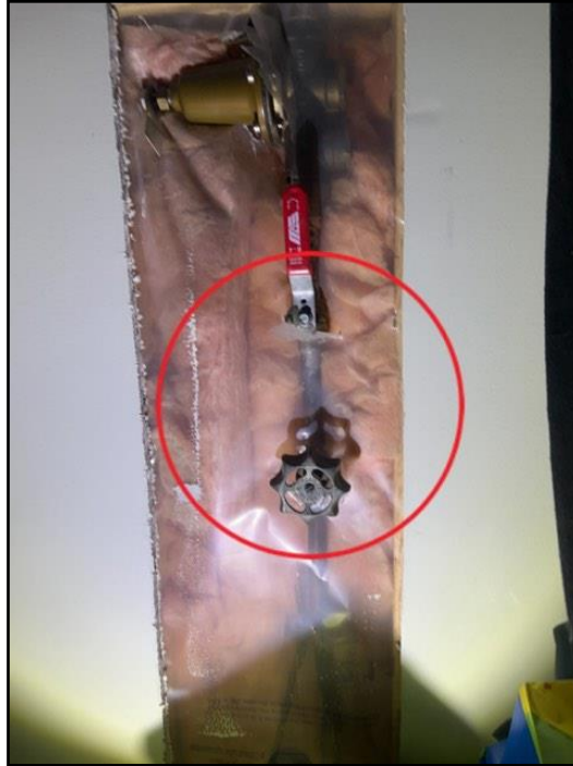
Water shut off
