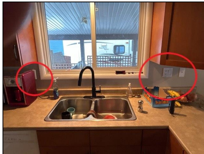
GFCI plugs missing
