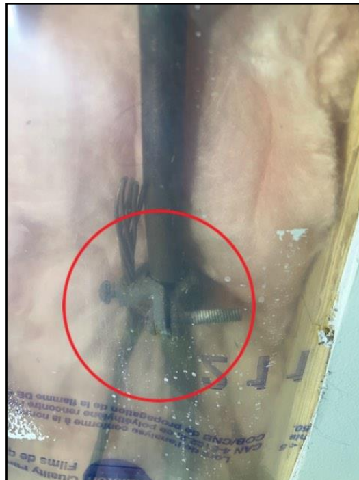
Copper - water pipe
