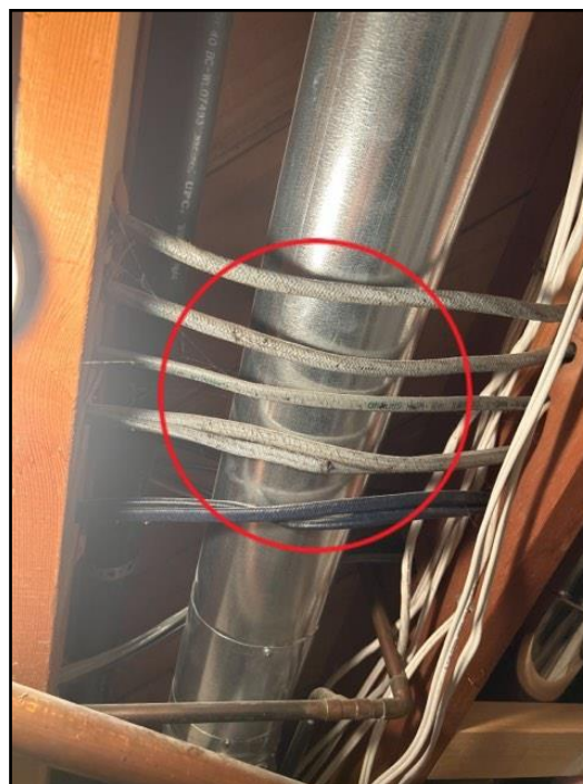
Wires touching ducts
