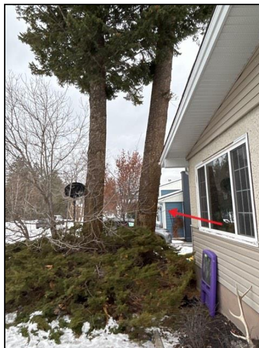
Trees too close to building
