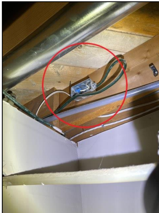
For junction box is missing
