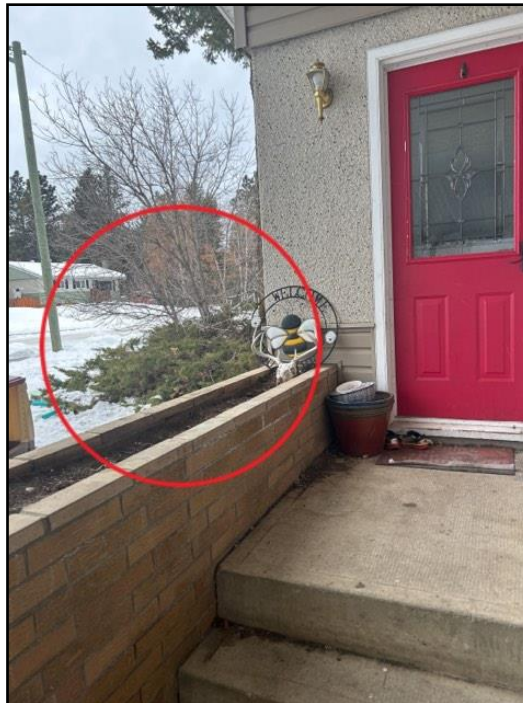
Missing guard rail
