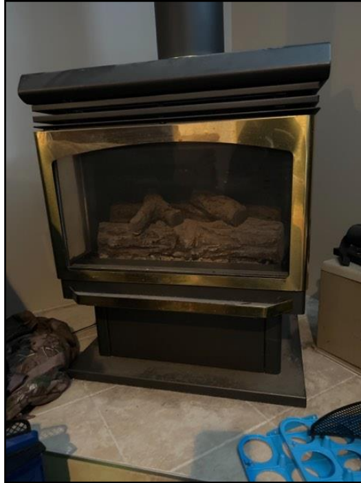
System was shut off
