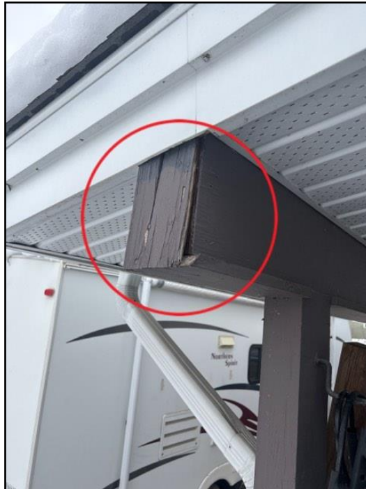
Paint - deteriorated / missing
